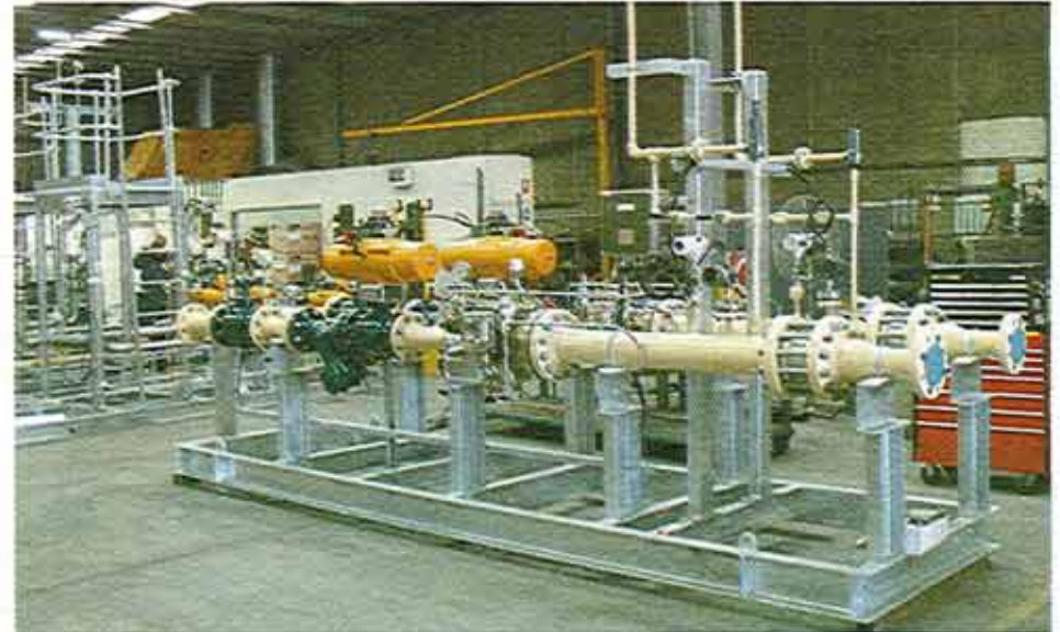
Above: Dual Pressure Let Down Skid
