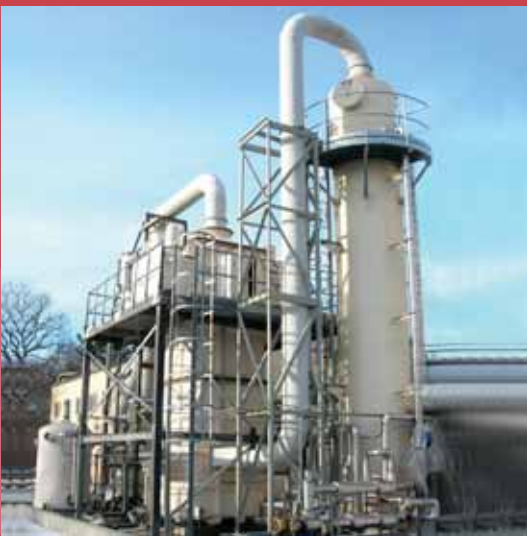
Above: Rota Bed® Turnkey Scrubber system.
